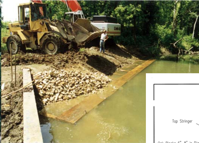
Lunker structure installation in progress. Trail Creek at I-94, Michigan City, Indiana
